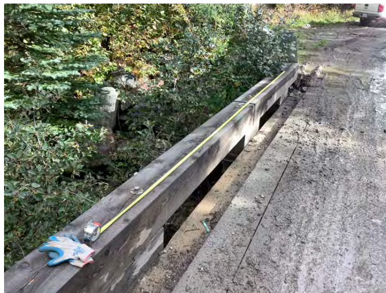
Guard Rail - need to replace with continuous riser due to poor quality tie riser connection
